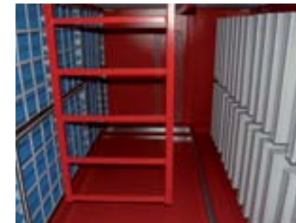
Right: View into filter house for gas turbine generator set GPB80 of KAWASAKI Gas Turbine Europe
