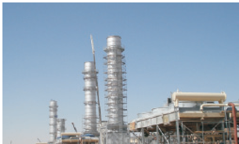
Saudi Electricity PP 9 – 12 units General Electric Frame 7EA Simple Cycle Exhaust Systems
