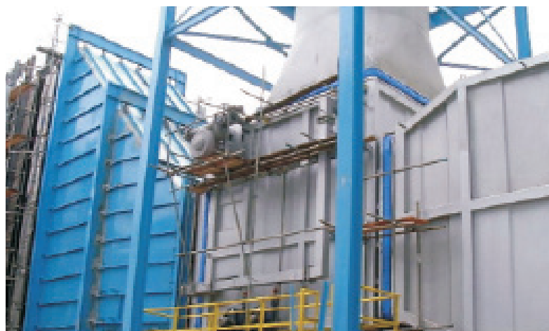
NUR Kulim High Tech Park – 4 Units General Electric Frame 6B Combined Cycle Exhaust Systems
